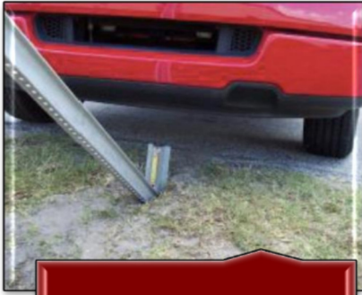
Breakaway Sign Posts
